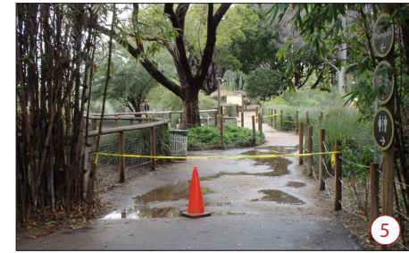
ERODED DIRT PATHS
